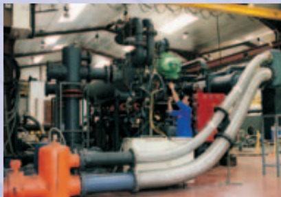
CIAT R&I Centre test bed
