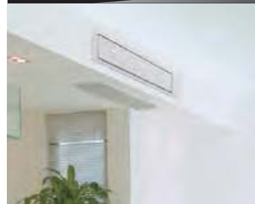
Bulkhead & Slim Duct
